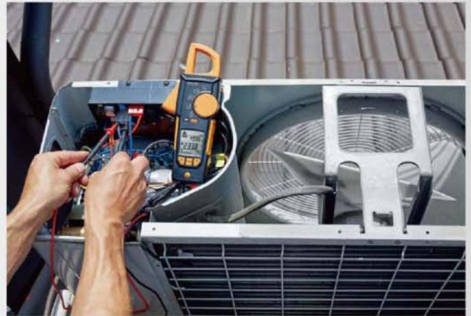
测量空调外机电压
